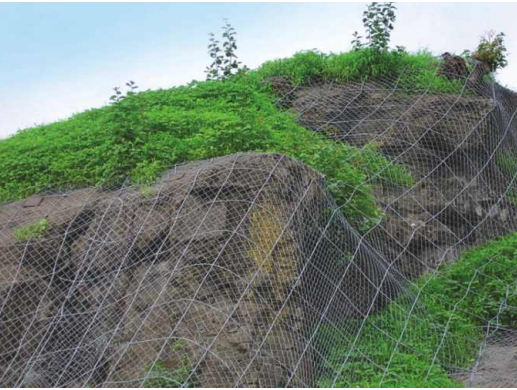
Rock Fall Protection Net
